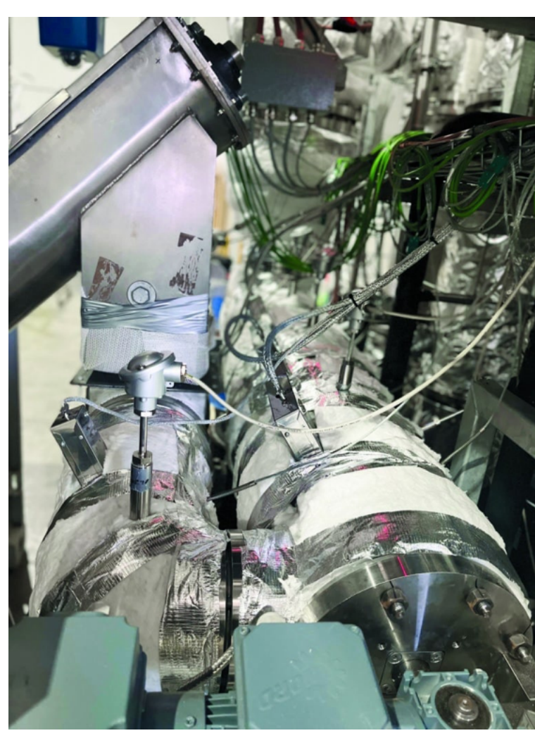
The first machine installed at APR Plastics will be used to test the process.
